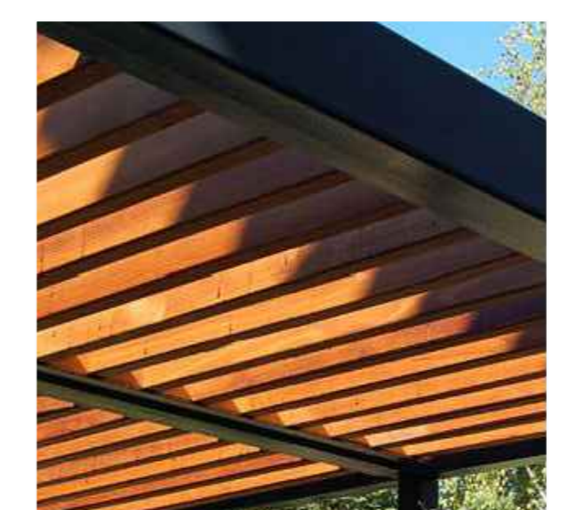
07 - vertical timber slat canopy set into dark grey metal frame to match glazing system
